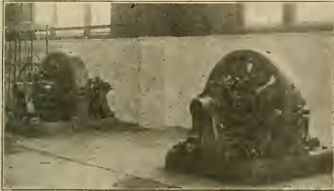
THE 150-K.W. ROTARY CONVERTERS SUPPLYING THE CRANE AND OTHER DIRECT-CURRENT MOTORS.
